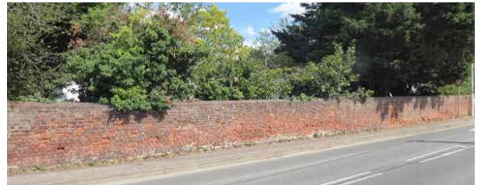
Figure 15 The brick wall, foliage and mature trees at the boundary of the former Braintree Campus of the Colchester Institute. The wall is to be rebuilt as part of application 19/01743/FUL, and the new wall is recommended for inclusion within the Conservation Area boundary
